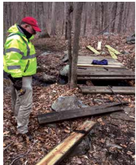
J. O'Brien at Bushy Hill Bridge to begin repairs. Photo by R. Helmecki.
