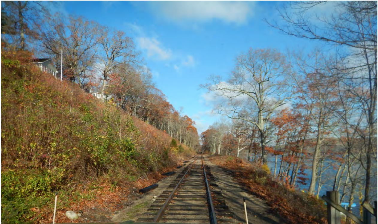
Looking North along corridor where track is being restored to FRA Class 1 (MP 12.9)
