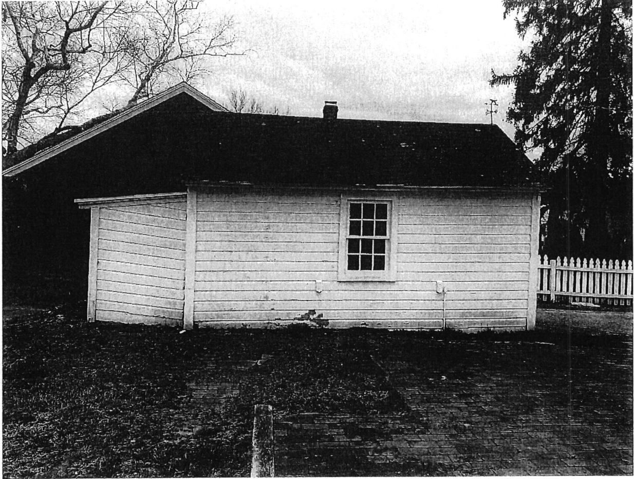
5 Scholes Lane garage showing settling.
