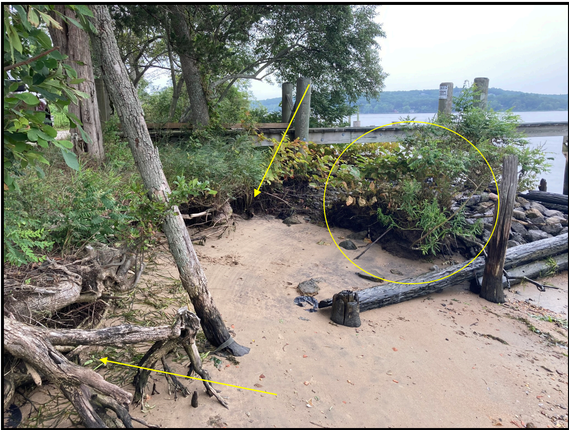
View of eroding shoreline and dislodged vegetation near boat launch area.
